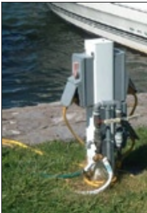
Water and electric service facility for boats.
